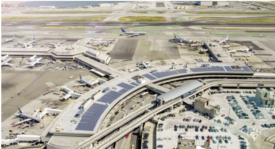
San Francisco International Airport Terminal 3 Rooftop Project America System Capacity: 450 KW
